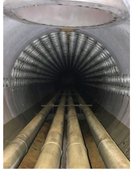
Figure 2: Boiler mud drum after cleaning
