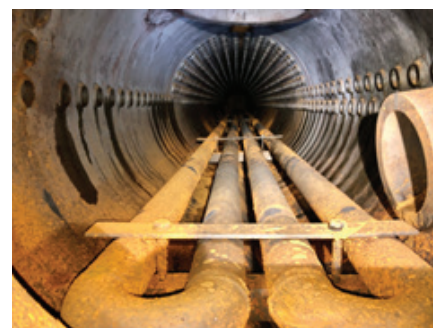
Figure 1: Boiler mud drum before cleaning
