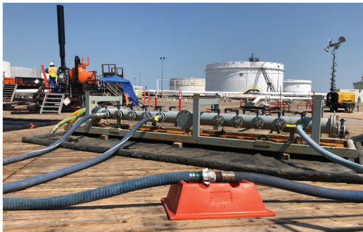
Figure 2: Tank Farm Manifolds
